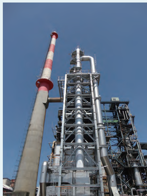
▲ Melamine heating furnace
